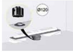
Drill the concrete with the help of drilling core for the pipe connection.
